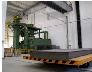
The steel in the VTS200 is shot blasted to create a clean painting surface
